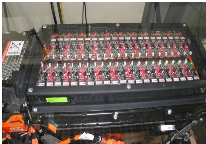
Ford C-Max Energi 8 kWh battery pack retrofitted with smart cell-level battery management technology
